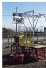
Beta Max Leo (VFD) Variable Speed 1000lb/2000lb Hoist on a Hydro Mobile mast climbing work platform.
